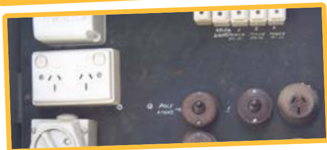
Zelemite backing board to an external switchboard
